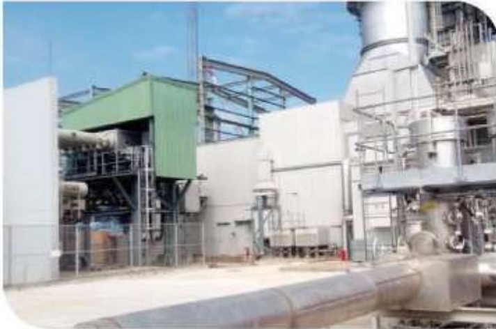
Kushlara Power Plant - a project by Pubali Bank Limited Principal Branch, Dhaka
